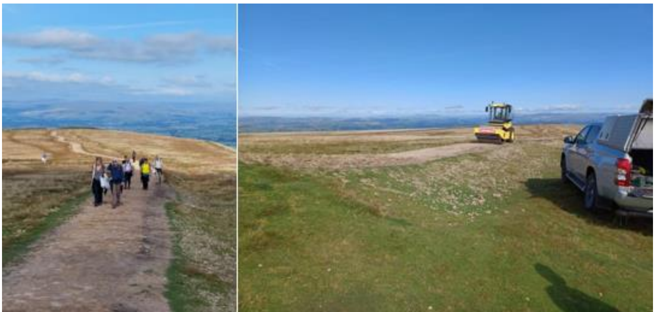
Regrading the subsoil path on Pendle summit to make it resilient after the increase in visitors post COVID and storms
