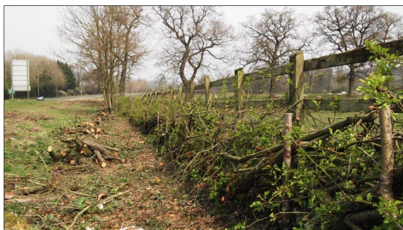
Coppiced and re-planted hedge at Old Hall, Roughlee (top); and newly laid hedge at Smithies Bridge, Chatburn
