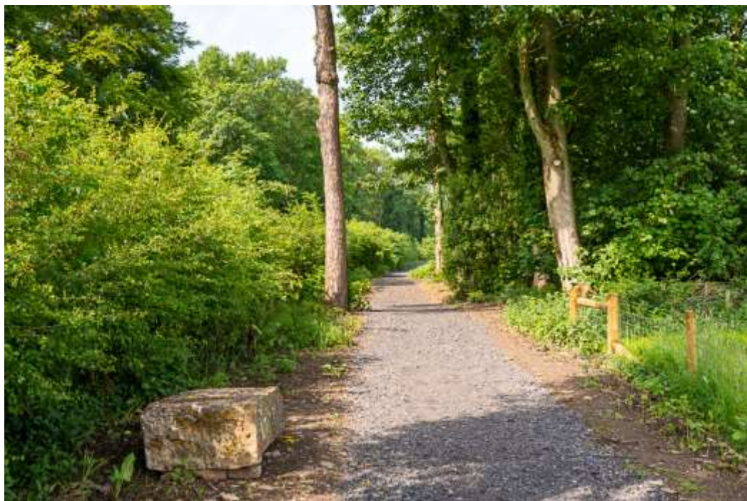
The completed bridleway, showing the newly planted hedge and seat for walkers and riders
