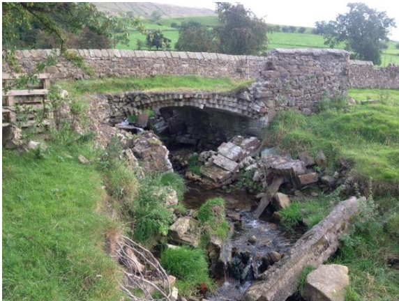
Route 9: GR SD 773 417 Collapsed Bridge, requiring replacement or repair
