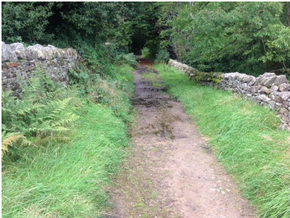
Route 2: Surface water due to insufficient/blocked drainage
