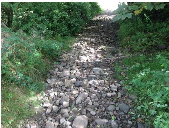
Route 2: Incline from Barley towards Roughlee. Eroded surface
