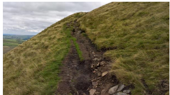
Route 7: Unpaved Section GR 805 409 patch repairs and drainage required
