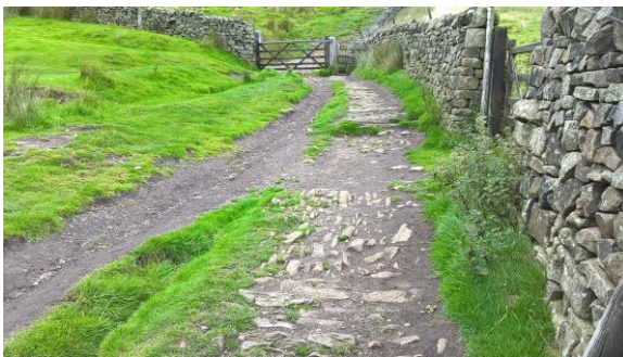
Route 7: Pendle Hill paved path repairs to Lower section required
