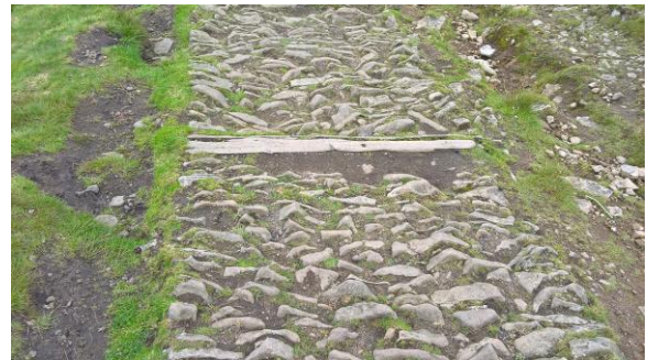
Route 7: Pendle Hill pitched path patch repair required (GR 807 414)
